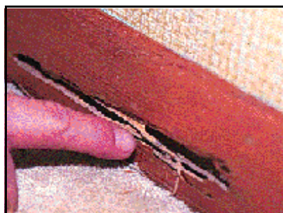
TERMITE DAMAGE TO BASEBOARD. HIDDEN INFESTATION WAS DISCOVERED WHEN VACUUM CLEANER ATTACHMENT PENETRATED SURFACE OF BASEBOARD. (M. Potter, University of Kentucky Entomology)
