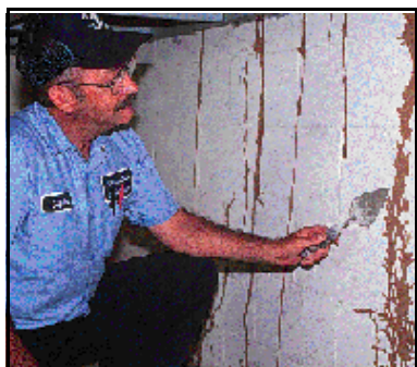
MUD SHELTER TUBES ON WALL (another indication of termite activity).
